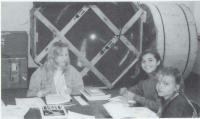
TOP: This is a look at the telecommunication room from the student's point of view.
